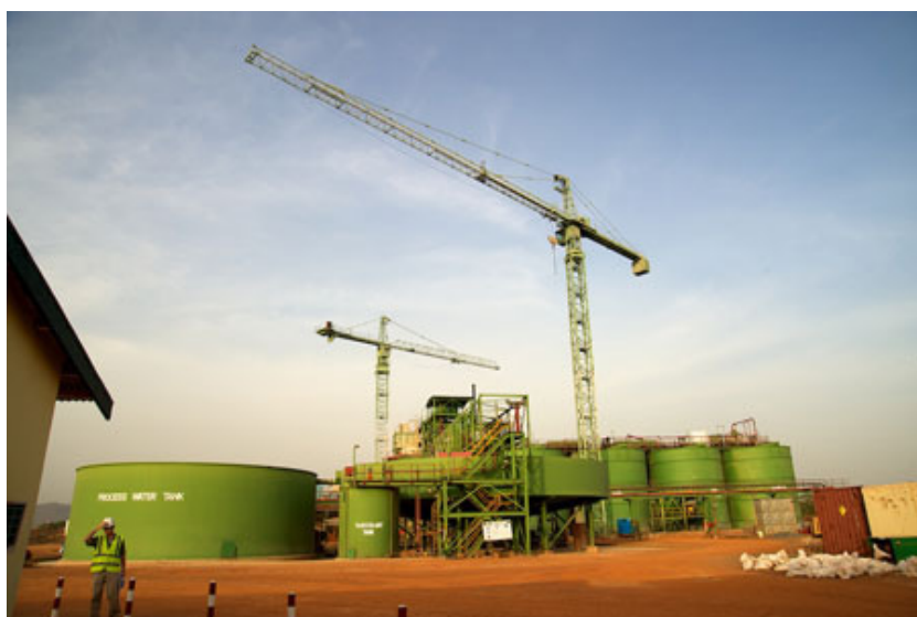
The Tabakoto gold mine plant. Bought in 2008, now up and running and pouring gold at $462/oz. That's COO Bradfield, to the left.
